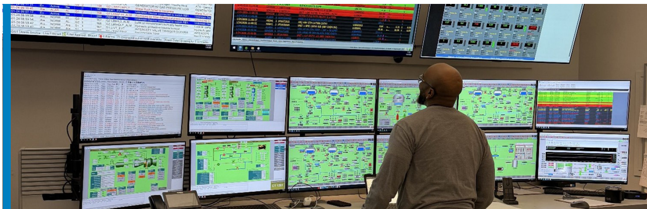
Photo: Earl McLean, Linden Control Room Operator, at the Block 1 Control Room Workstation.
