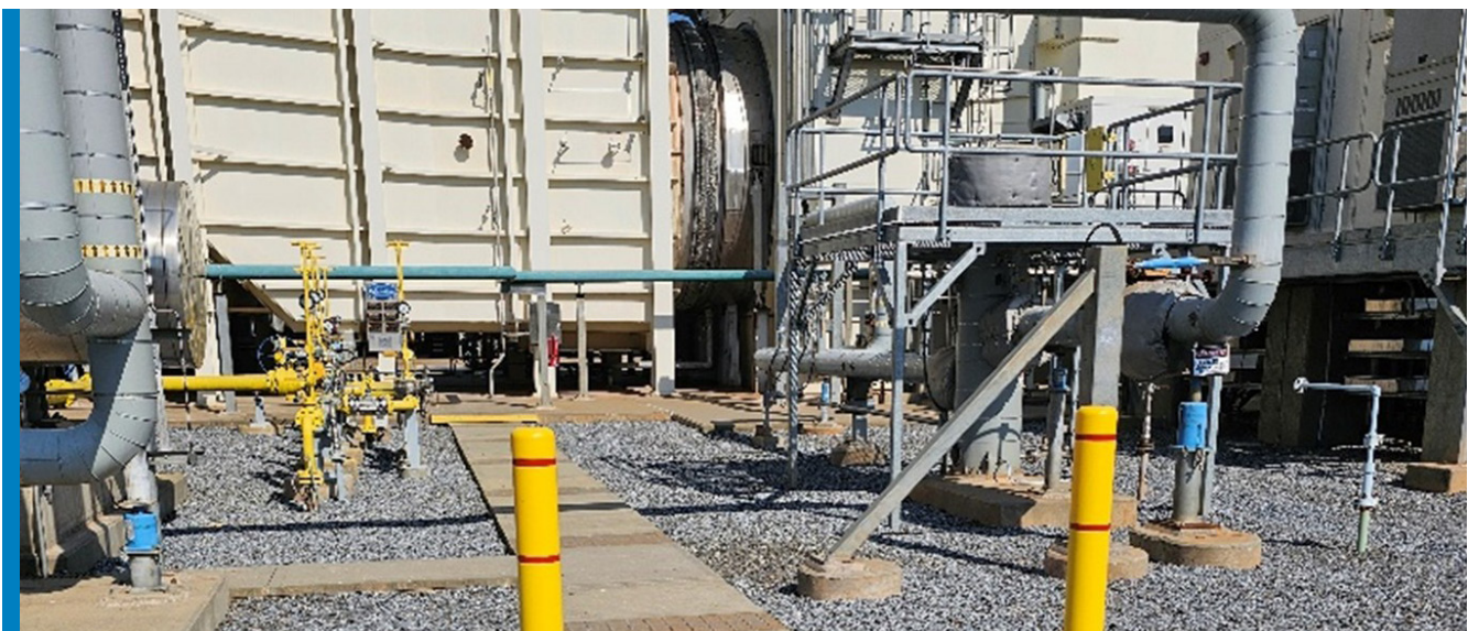
Photo: Kings Mountain Energy Center – Protective Bollards on Concrete Pads
